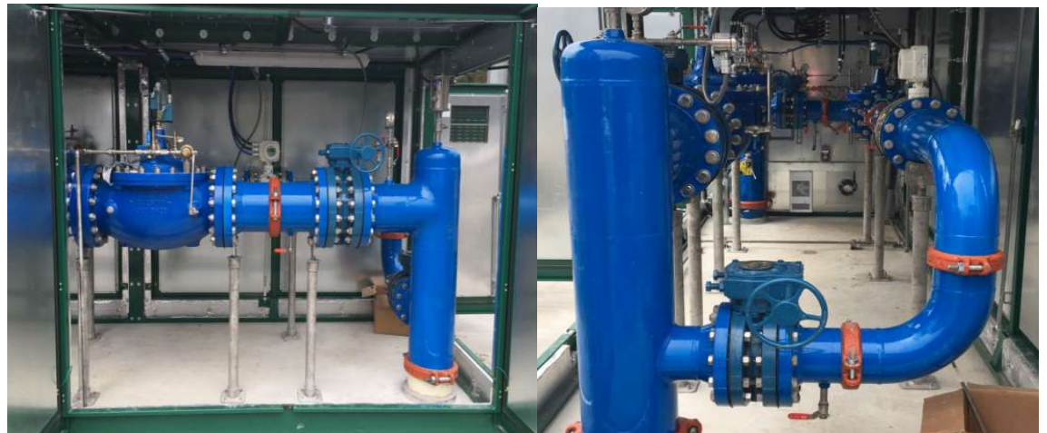
Figure 12: Norum Road PRV Station
