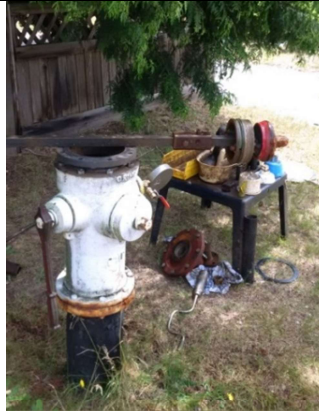
Figure 15: Fire Hydrant Undergoing Regular Annual Maintenance
